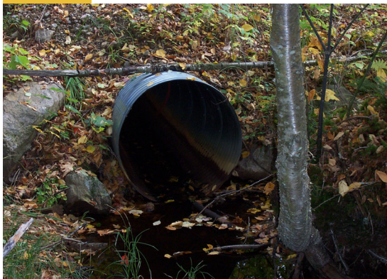
An example of an active culvert installation
