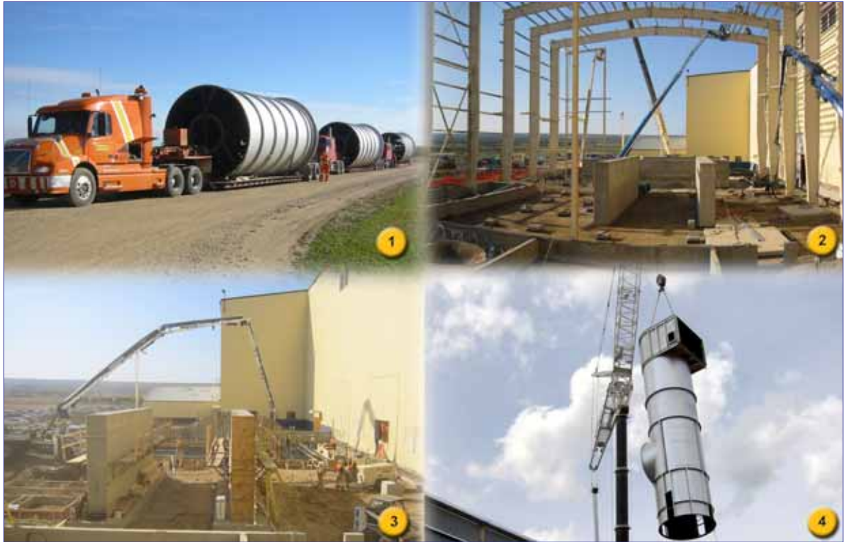
New dryers arriving on site (1) and various stages of wet fuel burner construction (2-4).
